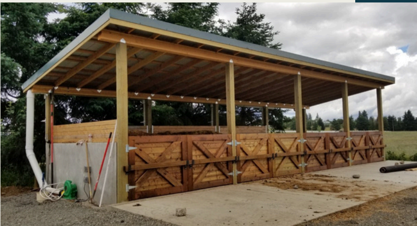
Covered multi-bin compost facility.
